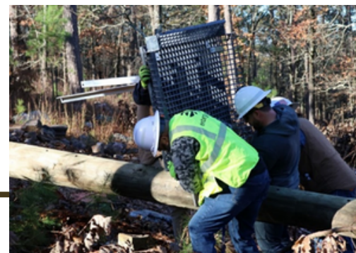
Top: Nesting platform placed by Entergy Arkansas at Lake Ouachita.
