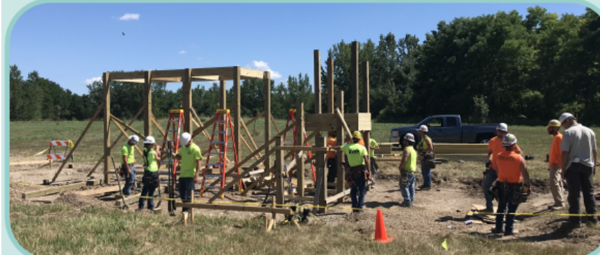
Volunteers work to construct an elevated shooting station at Saylorville Lake's archery range located in the Bob Shetler Recreation Area.
