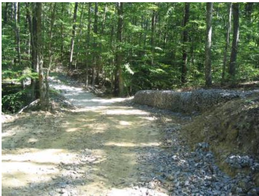
Figure 32. Cave Run Lake, KY. View looking north. Note the gabion placed for erosion control of the bank shown in Figure 27 (right side of the trail in this photo)
