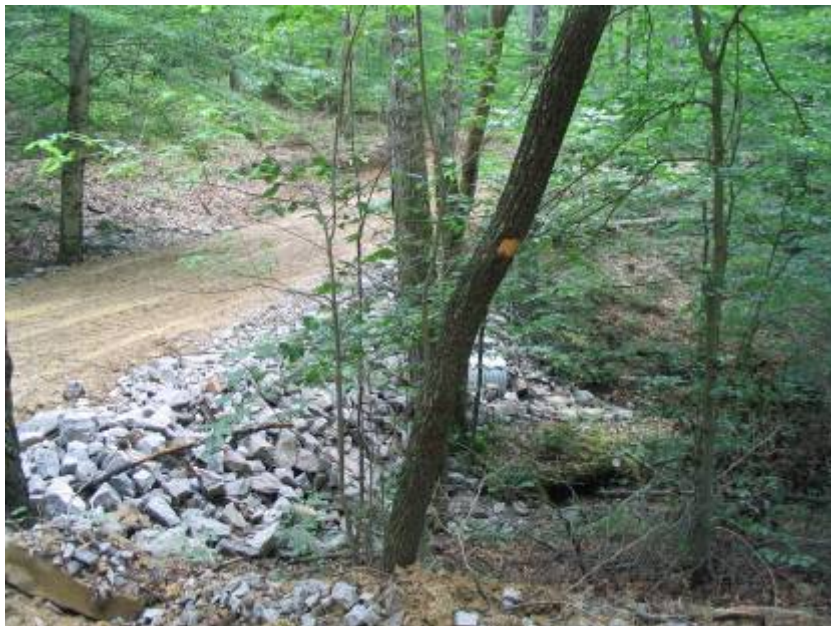
Figure 25. Cave Run Lake, KY. USFS's Sheltowee Trace Trail, July 2005. Culvert placed, with riprap on both sides of the trail where trail crosses drain
