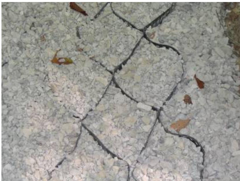
Figure 30. Cave Run Lake, KY. View of geocell after placement on the edge of a Sheltowee Trace section for erosion control
