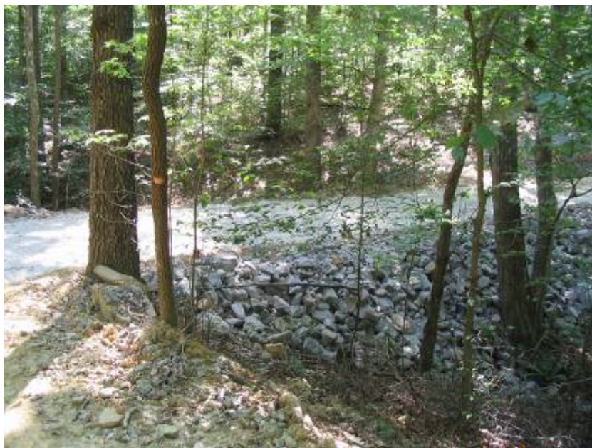
Figure 26. Cave Run Lake, KY. September 2005, view of finished section of trail that crosses drain shown in Figure 25. Tri-lock block has been placed, topped with gravel. USFS representative Loomis indicates this type of repair incorporating Tri-lock block and riprap "will last a lifetime"
