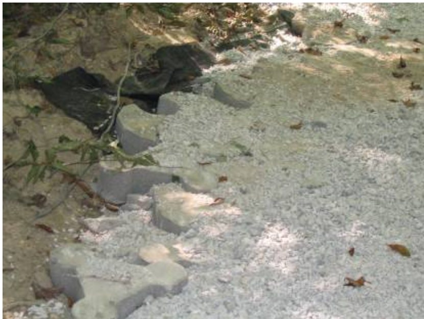
Figure 27. Cave Run Lake, KY. September 2005, view of rehabilitated section of Sheltowee Trace trail. The exposed trail edge shows materials used in the rehab: geotextile fabric underneath a layer of Tri-lock block, with top layer of gravel
