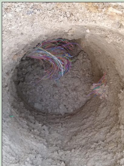
Digging without calling first often leads to damaged utility lines
