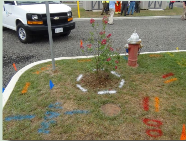
Arriving at the site after the utilities are marked will help you decide whether your dig location is safe or if you'll need to dig elsewhere
