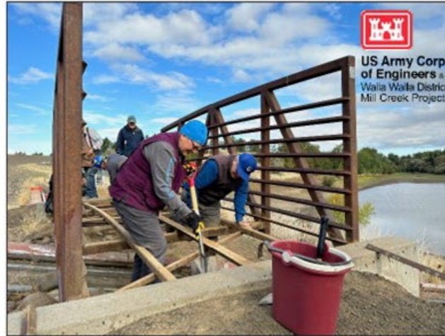
Above: Volunteers have removed the old wooden bridge surface and clean out around the exposing steel structure in preparation for the new boards.
