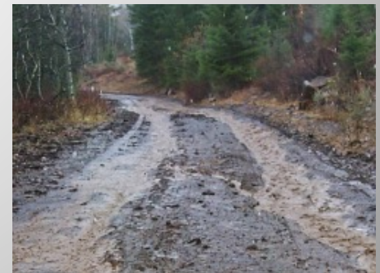
RATED – FAILED (1) F
