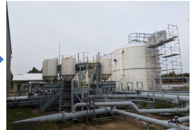
NanoBOT 7.5 HP-60 Treatment Technology as Installed at Montreal Pier Facility. Univ. Wisconsin LSRI/Great Waters Research Collaborative
