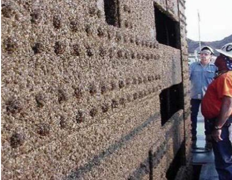
Figure 17. Quagga Mussels on the Davis Dam in California Source: Reclamation 2007
