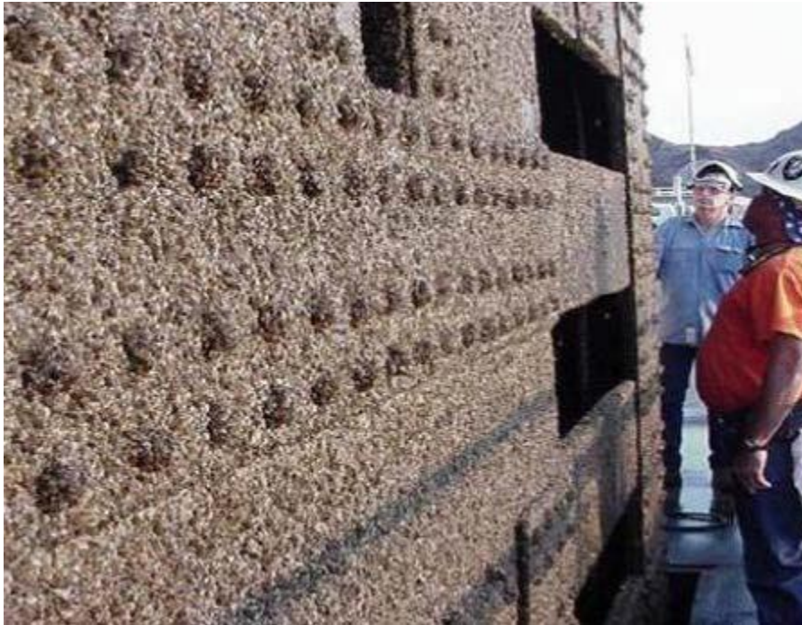
Figure 16. Quagga Mussels on the Davis Dam in California
