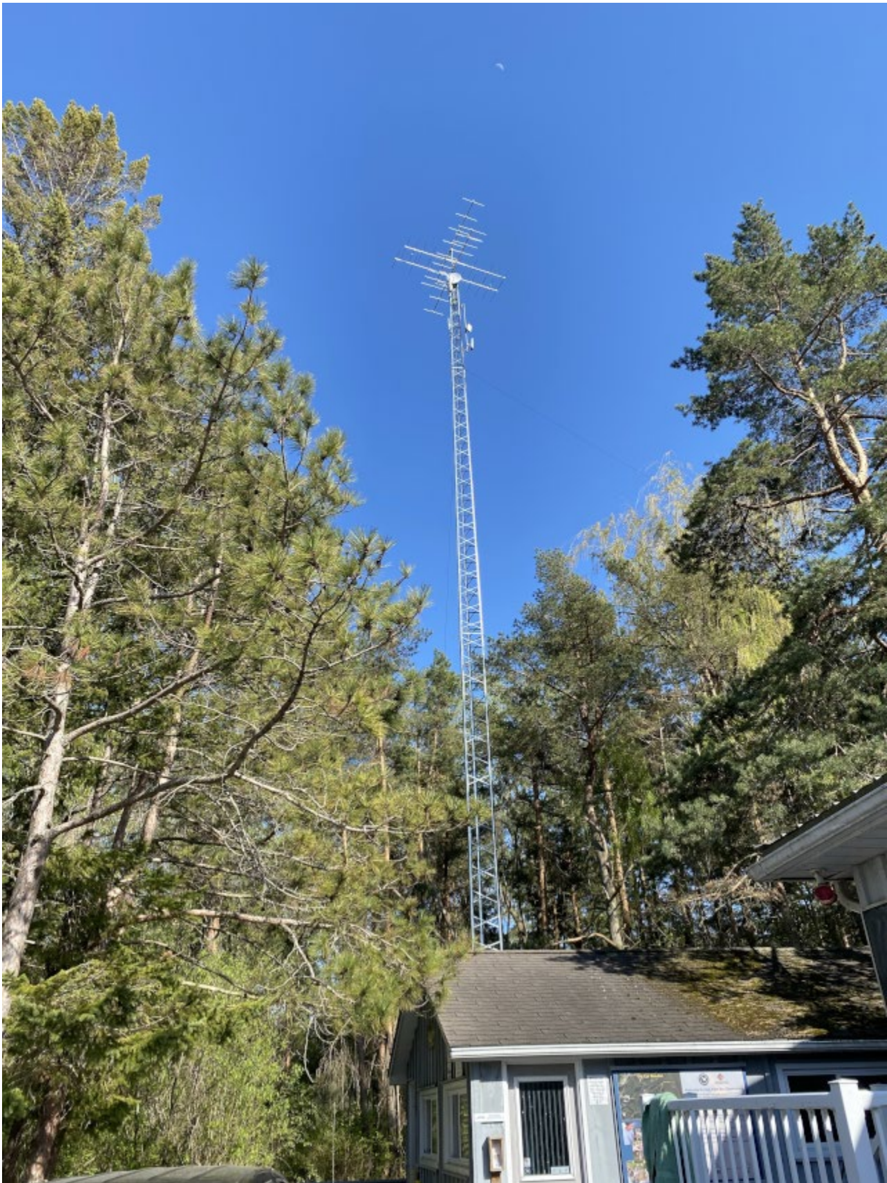
Figure 5) Motus antenna attached to existing tower.
