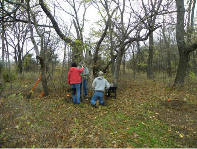
Volunteers Ken and Susan Johnson and Kenny Patterson team up to tackle installing 196 posts in the ground with Quikrete.
