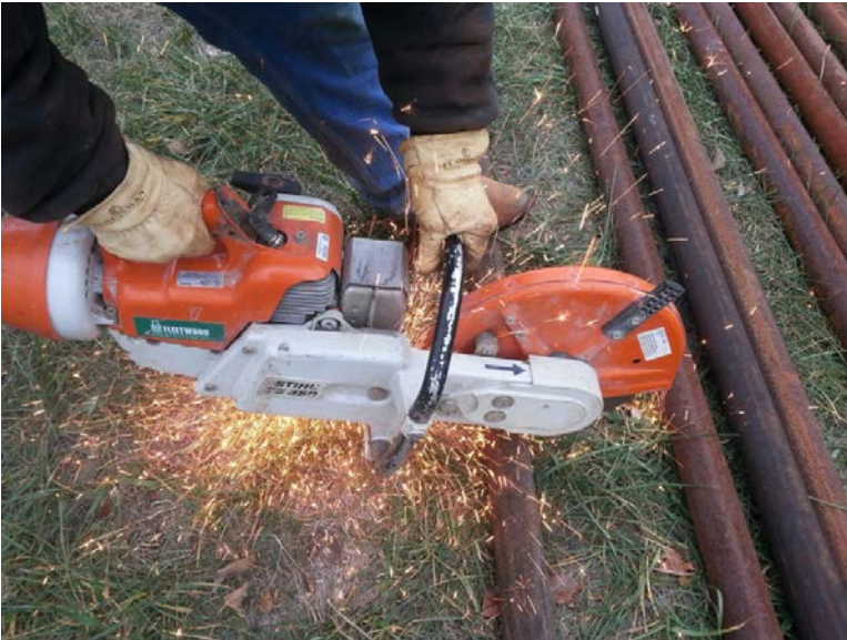
Volunteer Dale Mitchell cuts donated pipe to length for the perimeter fence uprights.
