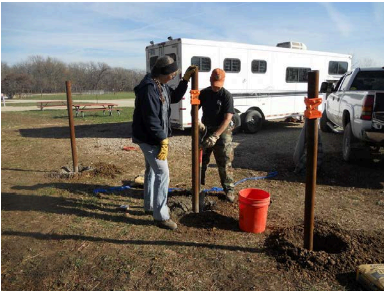
Volunteers Mary Mitchell (left) and Diana Skinner (right) ensure posts are level after placing Quikrete in the hole.
