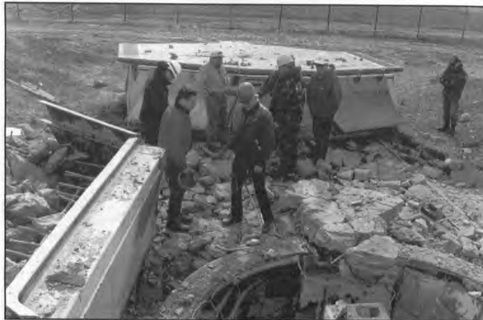
Corps and civilian workers inspect the results of blasting a missile silo. (Photo courtesy of Omaha District)
