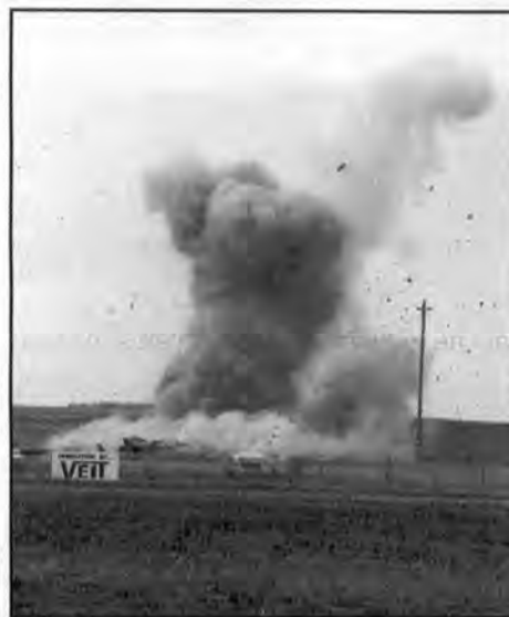
A cloud of smoke marks the destruction of an ICBM silo. (Photo courtesy of Omaha District)
