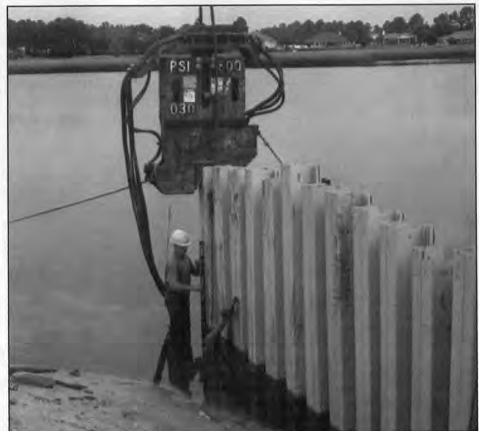
A construction worker drives vinyl sheet piling at a New Orleans District project. (Photo courtesy of New Orleans District)
