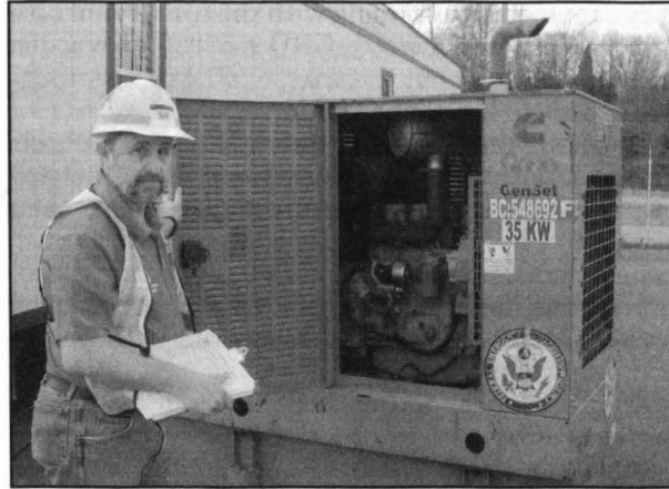
Charles Stroup with a generator similar to the ones he inspected during the ice storm. (Photo courtesy of Louisville District)
