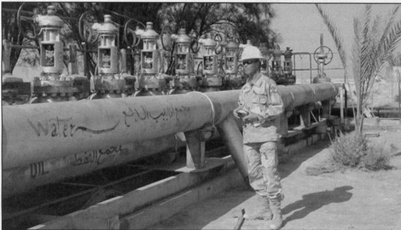
A Corps employee checks valve repairs at Cluster Pump Station 3 in the South Ramaila Oil Fields. Helping restore Iraqi oil production capacity is just one of the many missions of the new Gulf Region Division (Provisional). (U.S. Army Corps of Engineers Photo)
