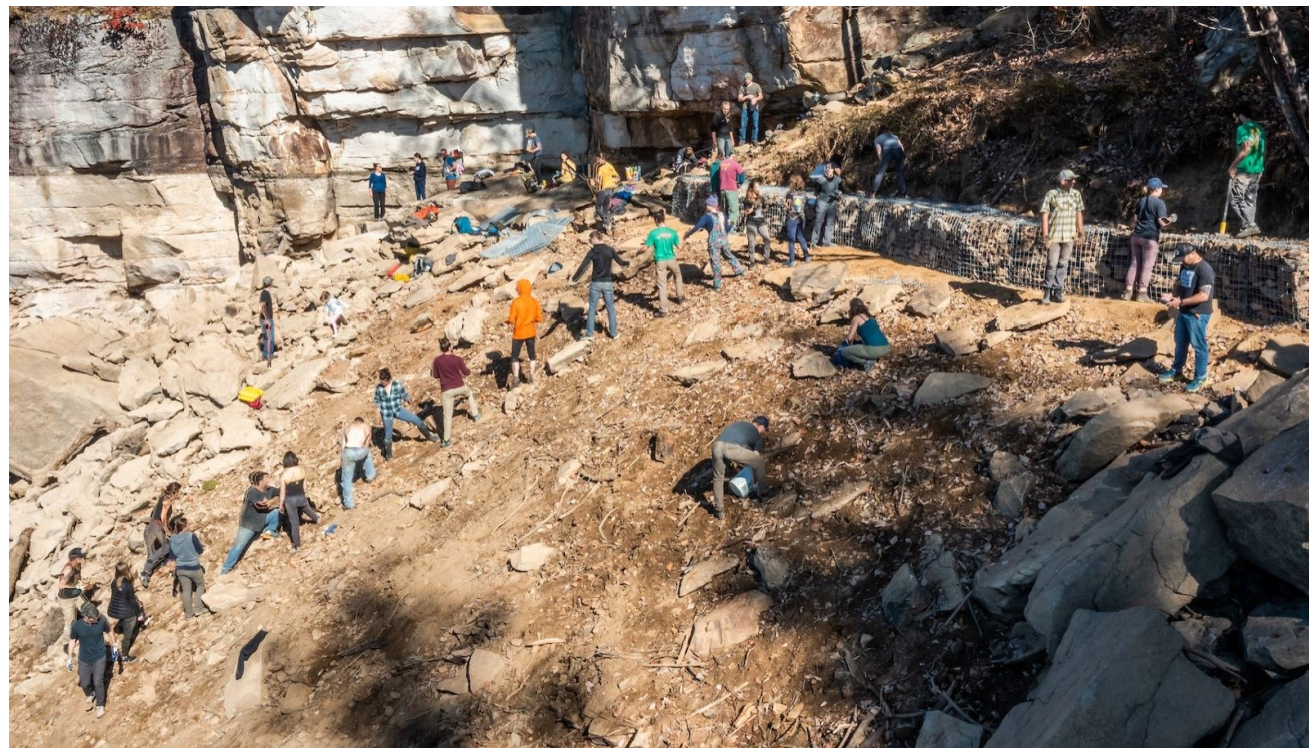
2022 Excellence in Partnerships Award Winner: New River Alliance of Climbers volunteer event constructing gabion baskets with barged-in equipment and materials. This partnership focused on mitigating impacts of and improving access to popular rock-climbing routes around Summersville Lake, WV.
