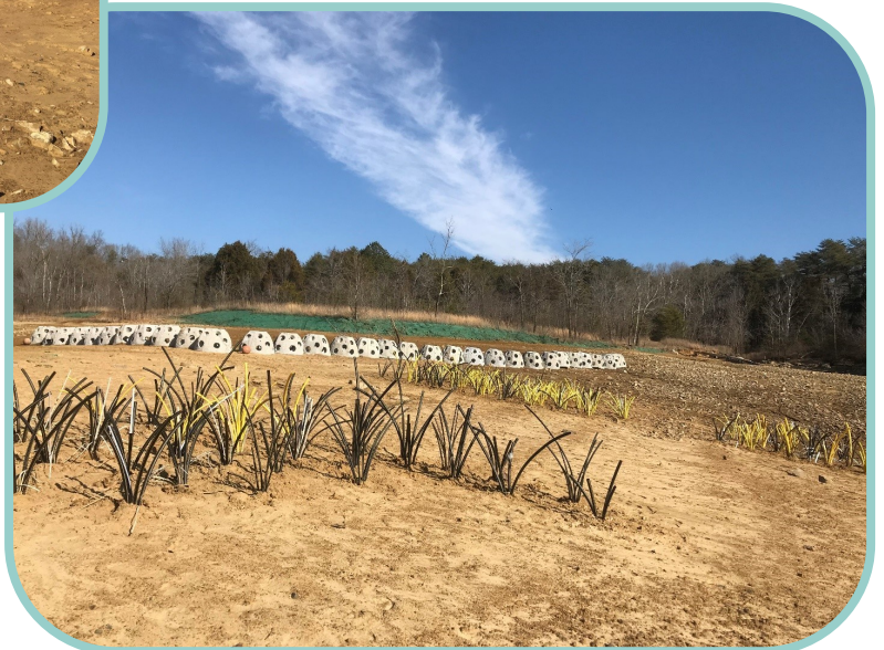
Site 2 of the Nolin River Lake Bank stabilization project showing pre and post-installation of reef balls, hydroseeded native grasses and wildflowers, and artificial fish attractors
