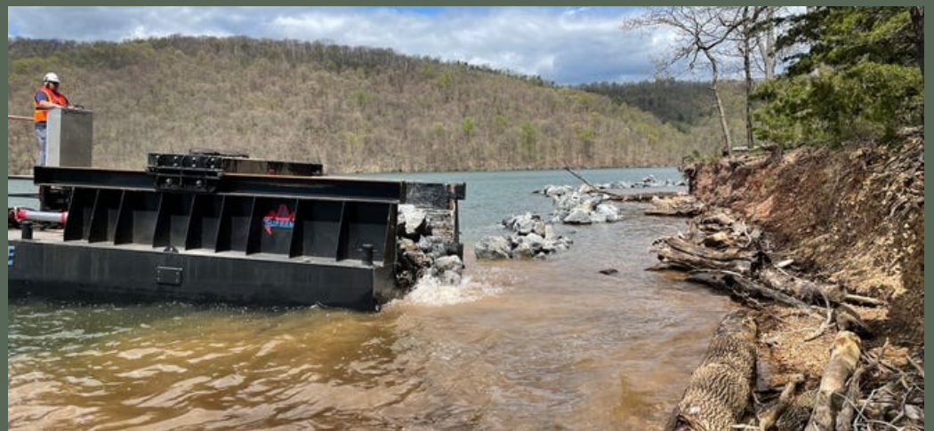
Photo above: Crews unload rocks along the shoreline of Raystown Lake to create better fishing habitat and reduce shoreline erosion. Photo provided by Ben Page, PAFBC.
