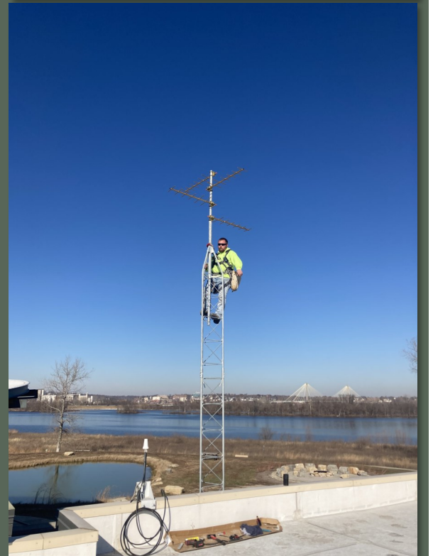
Photos Above: Installation of the MOTUS tower atop the Rivers Project Office in West Alton, MO.
